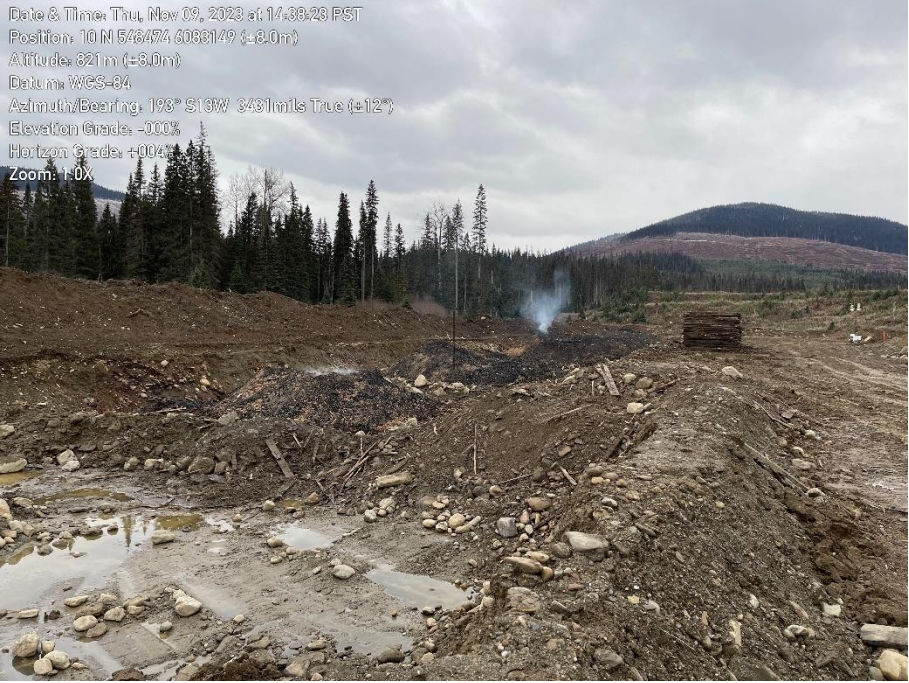
Photo 1. Burn piles observed by EAO CEB on November 9, 2023, near KP 166+100.
