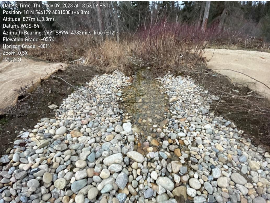
Photo 6. Watercourse number J234.99 looking downstream at the bottom end of the crossing.
