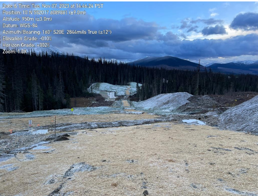
Photo 13. KP 151+100 approximately. Overview of RoW looking towards high-chain. Measures installed per the WEP.
