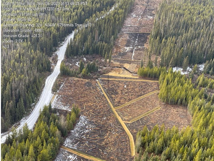
Photo 18. Overview of KP S_13 as seen from the air on November 8, 2023. Looking at the watercourse crossing at KP S_13+050. Final clean-up completed.
