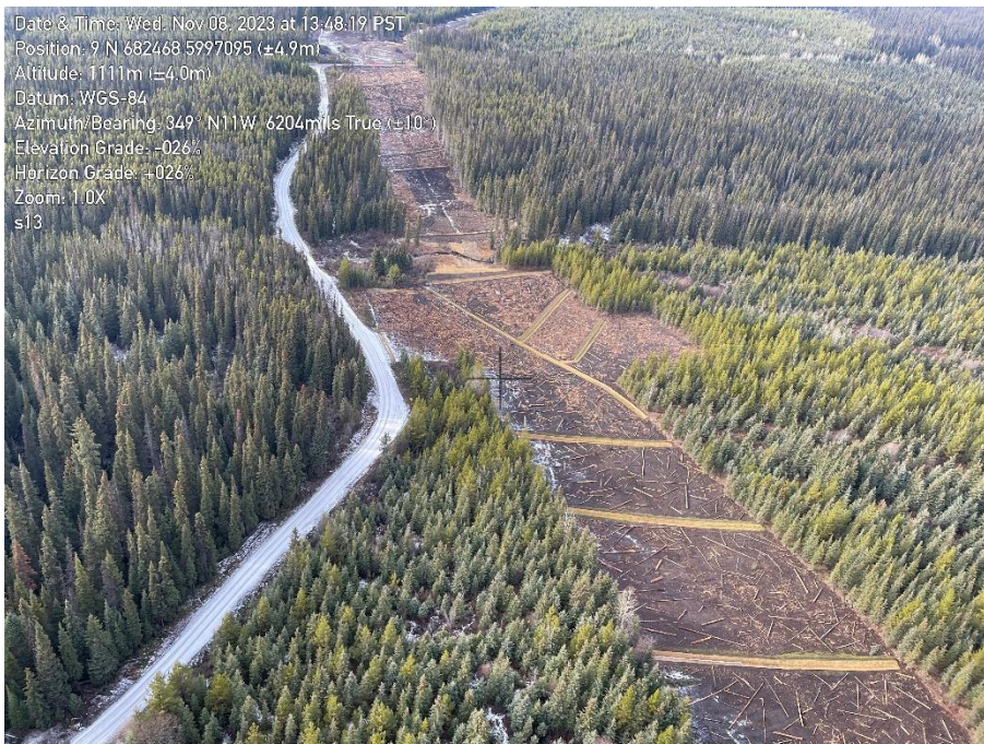
Photo 17. Overview of KP S_13 as seen from the air on November 8, 2023. Looking high chain towards KP S_13+050 watercourse crossing. Final clean-up completed.
