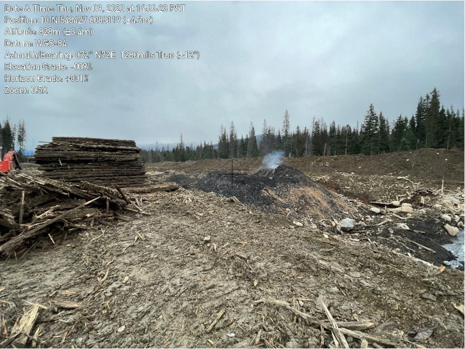
Photo 2. Burn piles observed by EAO CEB on November 9, 2023, near KP 166+100.
