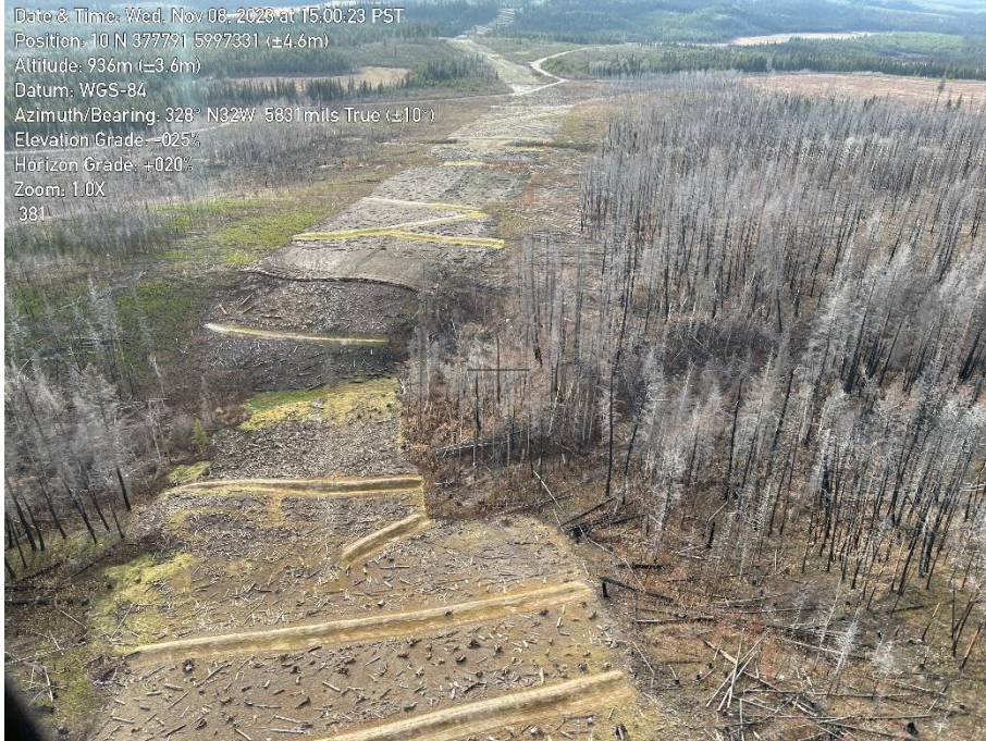
Photo 15. Overview of KP 381 as seen from the air on November 8, 2023. Final clean-up completed.
