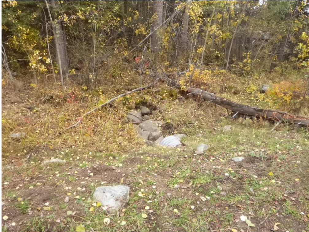
Photograph 7. Culvert across an access road in the Project area. Culvert was dry at the time of the site visit (September 29, 2021).
