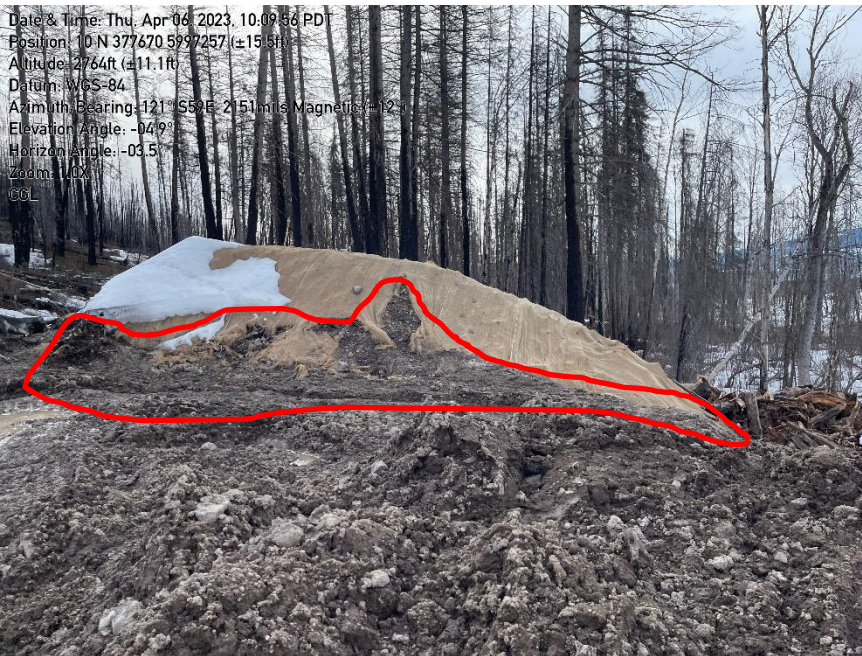
Photo 13: Soil stockpile cover in need of maintenance and missing straw wattles around base.
