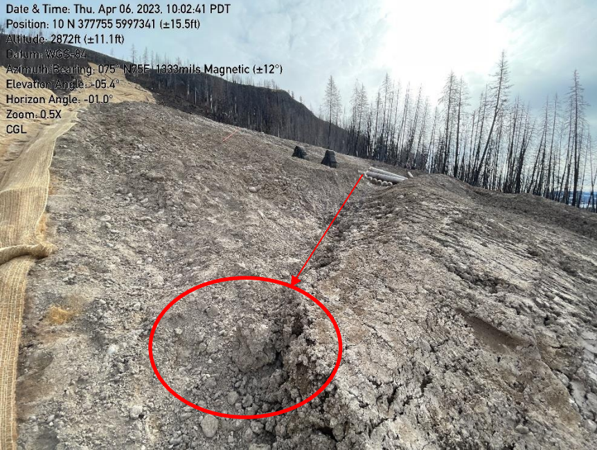
Photo 12: Cross ditch missing straw wattles and missing rock lined feature.
