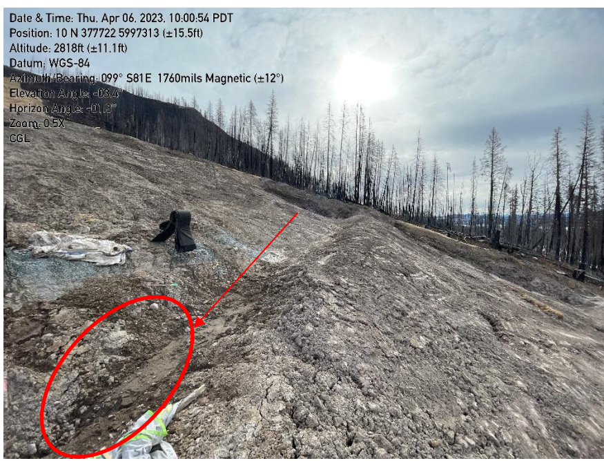
Photo 11: Cross ditch missing straw wattles and missing rock lined feature.
