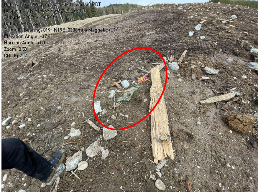
Photo 5: Fabric and plastic construction waste left on reclaimed ROW.
