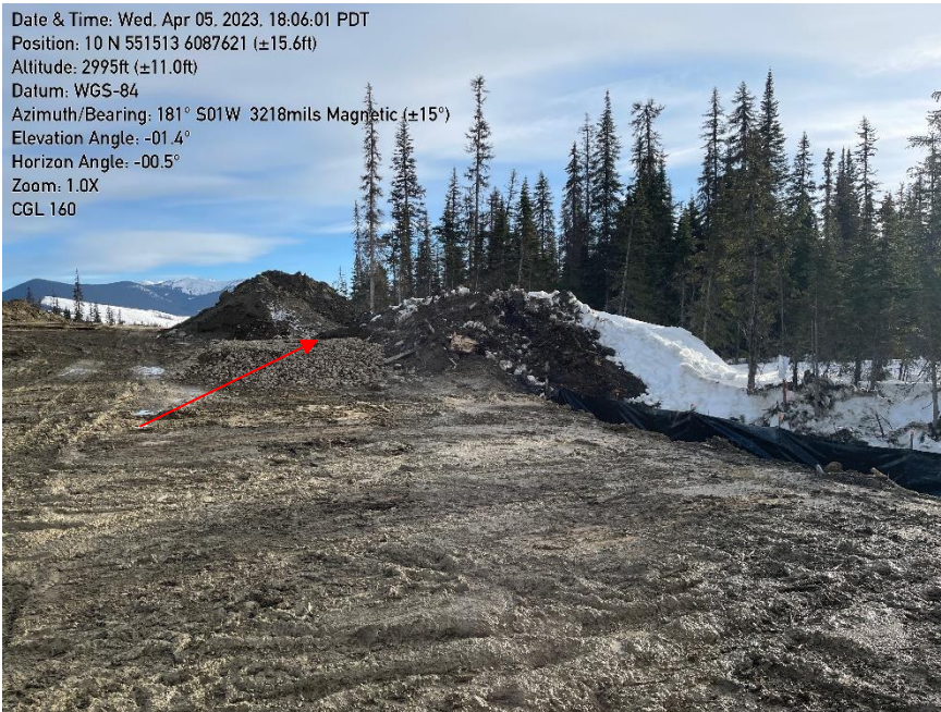
Photo 3: Gap in snow berm along ROW.
