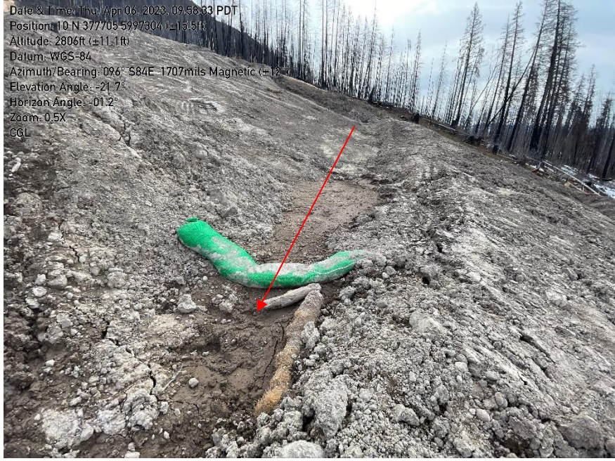
Photo 10: Cross ditch missing correctly installed straw wattles and missing rock lined feature.
