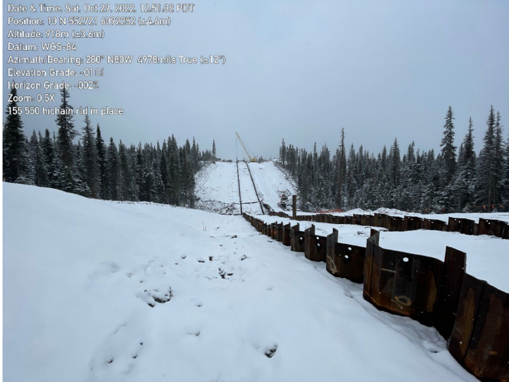
Photo 1: overview of sheet pile walls intercepting waterbars at approximately KP155+550, looking hichain. Waterbars do not penetrate the sheet pile with exception of lowermost waterbar on either side of watercourse and will not function as prescribed by the ESCP.
