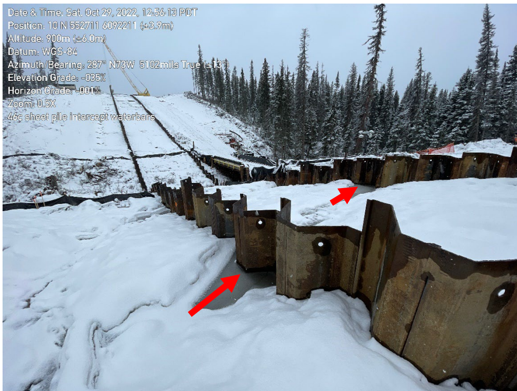
Photo 2: Sheet pile walls intercepting waterbar at approximately KP155+675. Note lack of opening in sheet pile wall.
