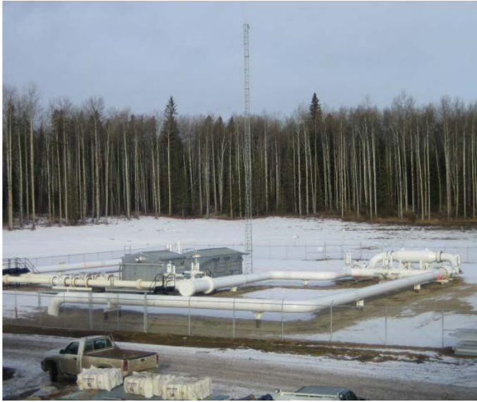
Figure 2-4: Typical meter station site
