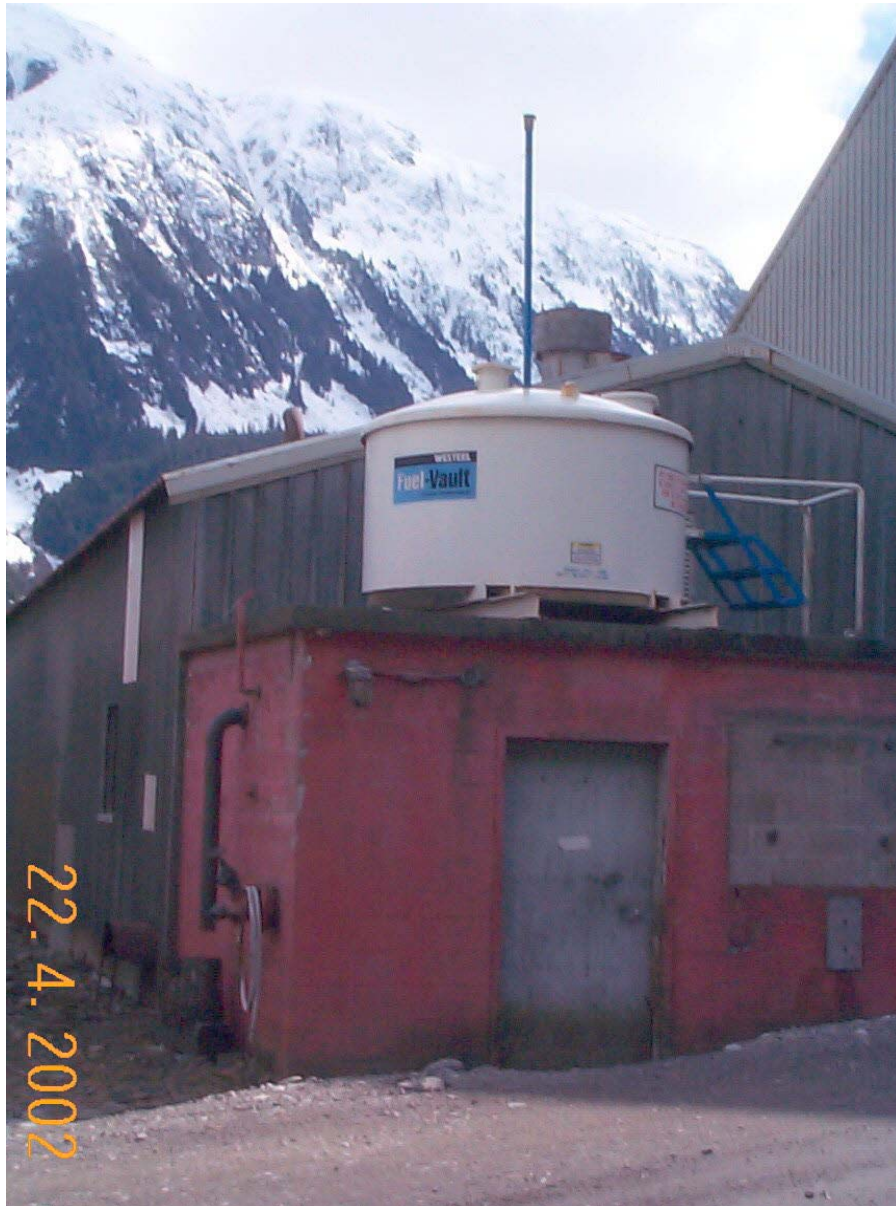
Spill-Proof Fuel Storage Tank on Wharf Site
