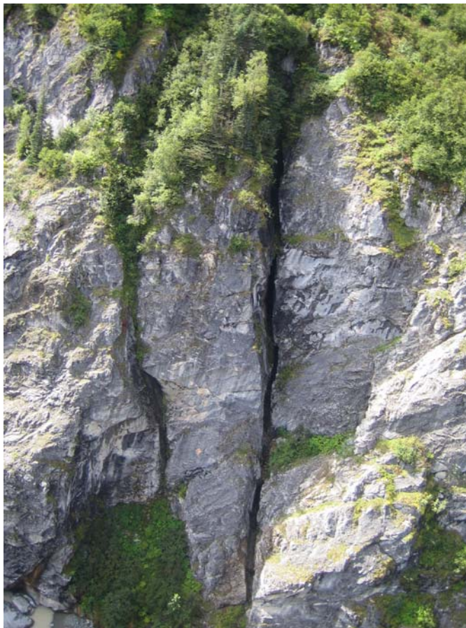
Photo 2. Joint in limestone with solution widening. October 2006
