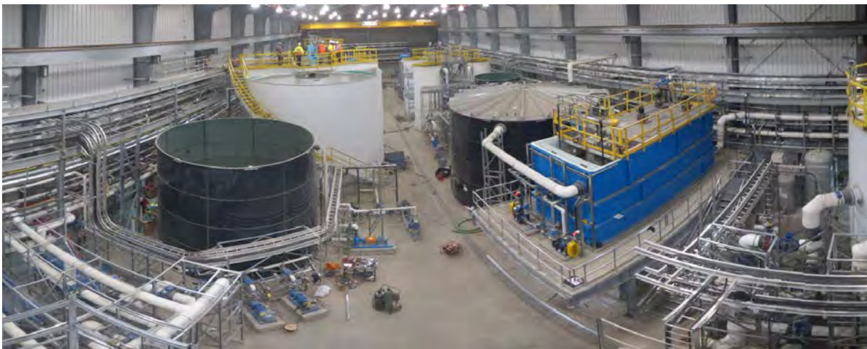
Figure 6-5. West Line Creek Active Water Treatment Facility, April 2014.
