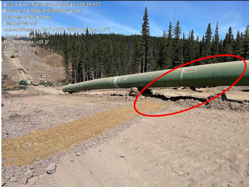
Photo 4. Lined ditch at KP 567+050 not installed to depth specification and unlined across a portion of the ROW.
