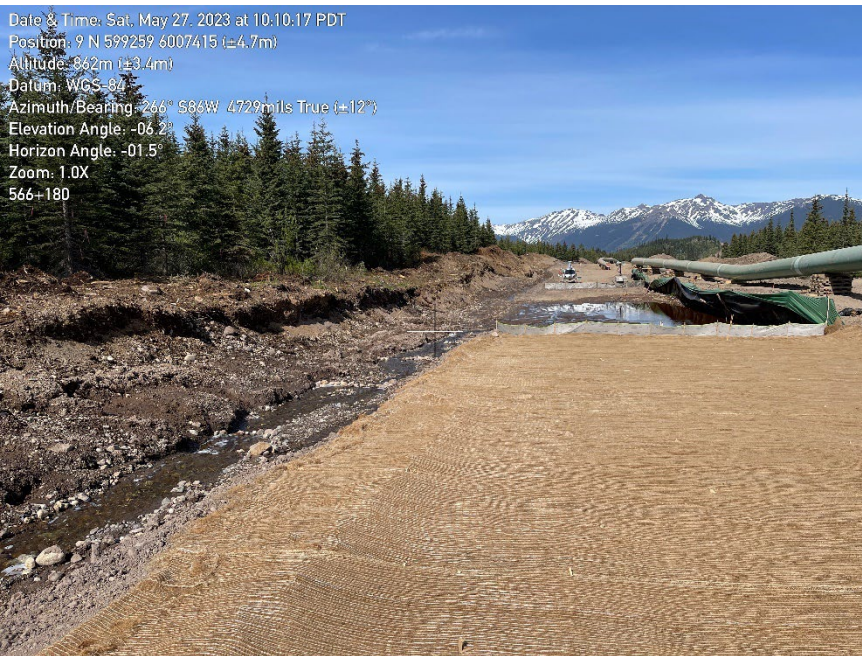
Photo 2. Cleared portion of ESIW WET-566.3 utilized as a catchment area for unlined ditches at KP 566+200. The WEP specifies that the wetland be delineated from the ROW.
