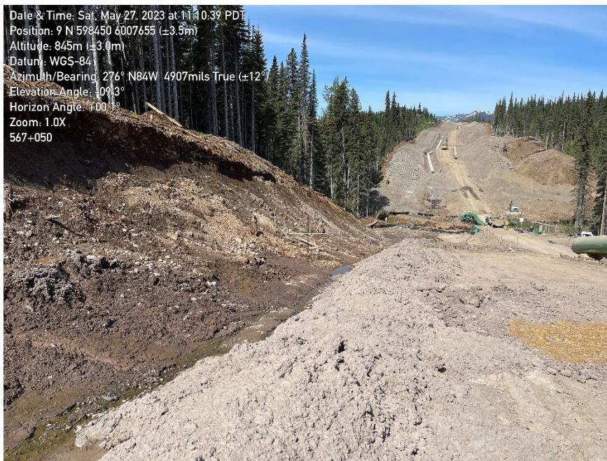
Photo 5. Ditch at KP 567+000 and 567+080 not lined as specified in WEP.
