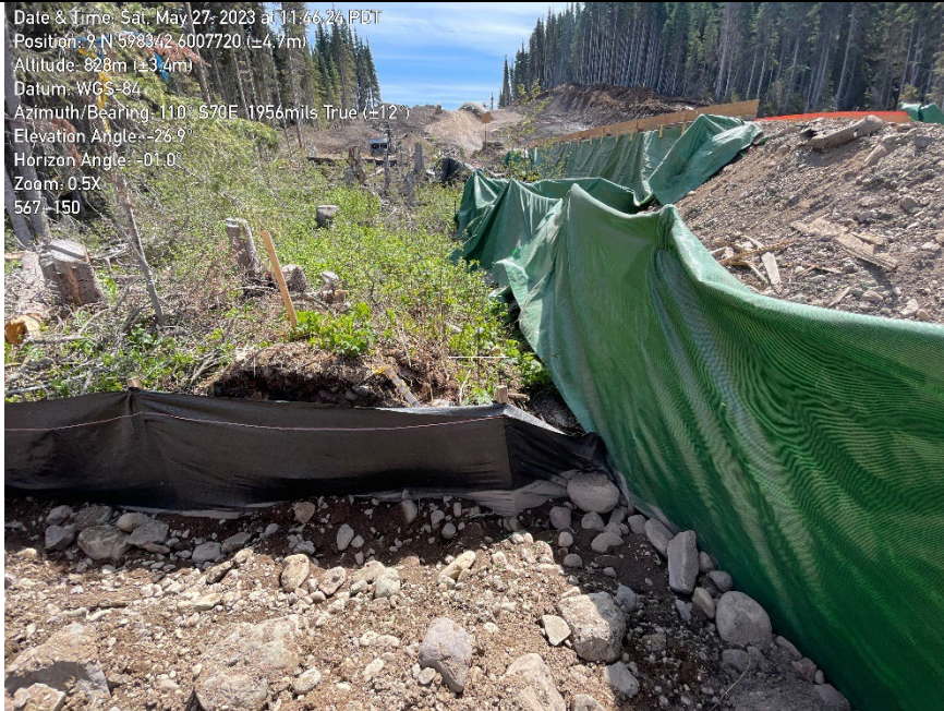
Photo 6. Gap in the corner of sediment fencing at KP 567+150 where evidence of sediment movement was observed.
