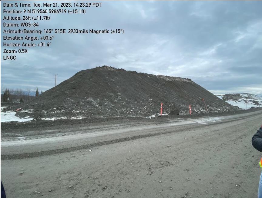
Photo 11: Snow pile located beside stockpile with perimeter ditch.
