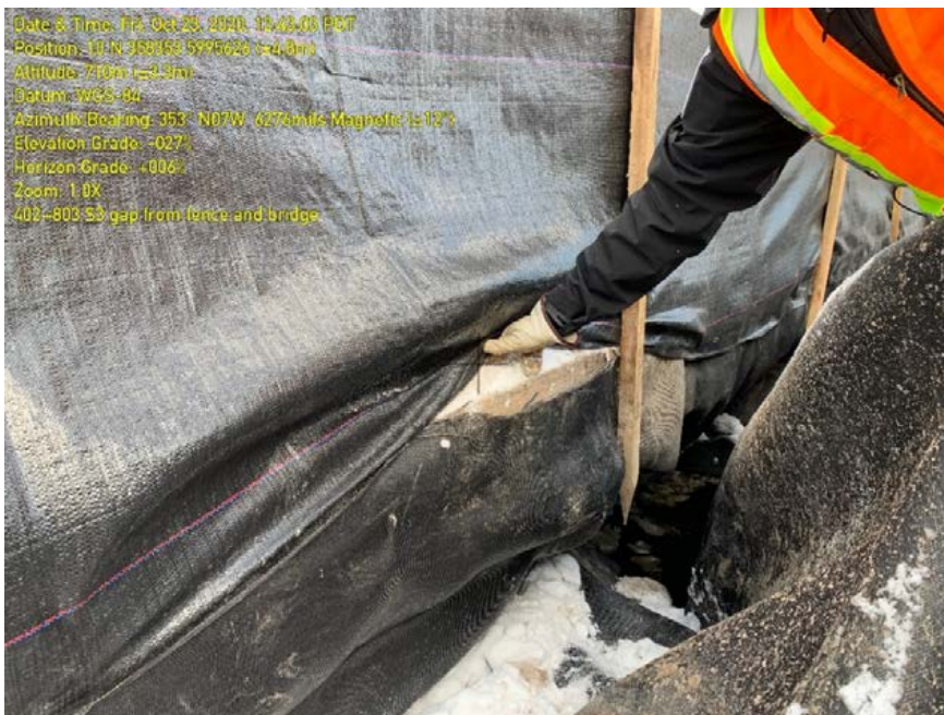
Photo 30: Sediment fence stapled to bridge over S3 stream. Ineffective installation.
