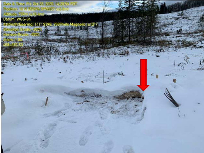
Photo 55: Work package 3. Straw rolls not keyed into place correctly. Gap beneath roll allowing water to flow beneath measure.
