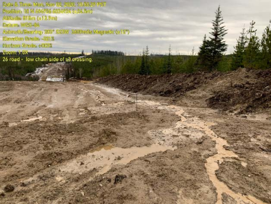
Photo 69: Exposed surface materials from stripping of right of way, active erosion. Sediment mobilizing towards watercourse #WC272.
