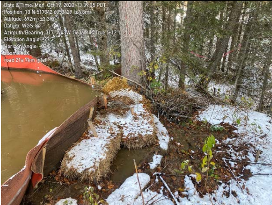
Photo 23: Sediment fence installed across water feature and overwhelmed. Straw bails installed incorrectly. Sediment laden water discharging towards Crooked River downslope of site.
