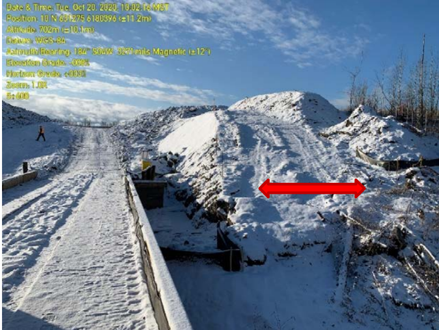
Photo 21: Discontinuous sediment fencing adjacent to fish-bearing stream feature.
