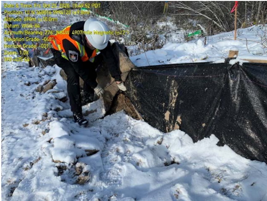
Photo 32: Sediment fence not attached to geotextile, large gap. S4 in background.
