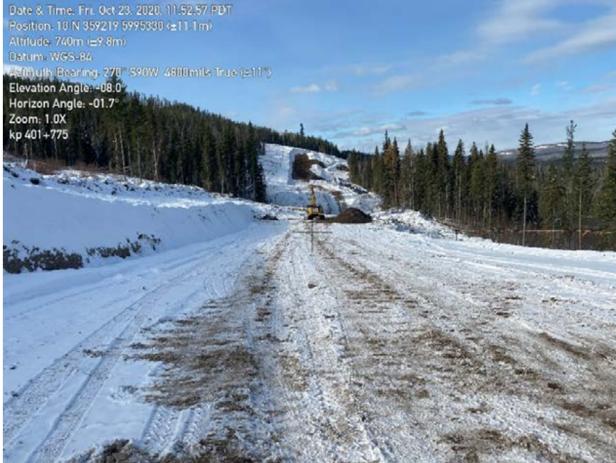
Photo 3: Exposed right of way near KP402. Lack of winterization on right of way through this portion of the Project.
