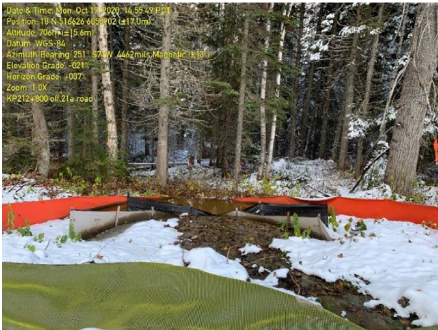
Photo 24: Sediment fence across channel at culvert outlet on 21a road. Fencing overwhelmed, not maintained and sediment laden water discharging off site.
