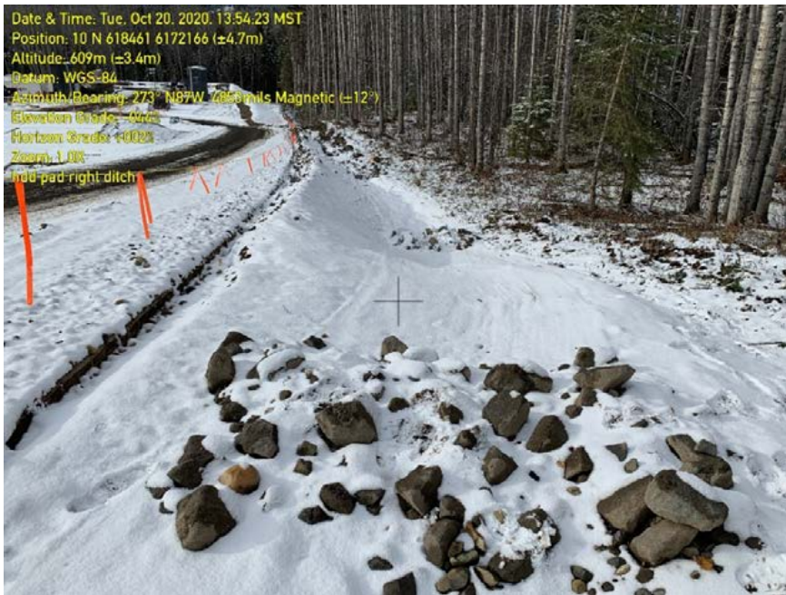
Photo 13: Drainage ditch on right side of Murray HDD pad. Check dams discontinuous and not installed to specification. Note coarse material.
