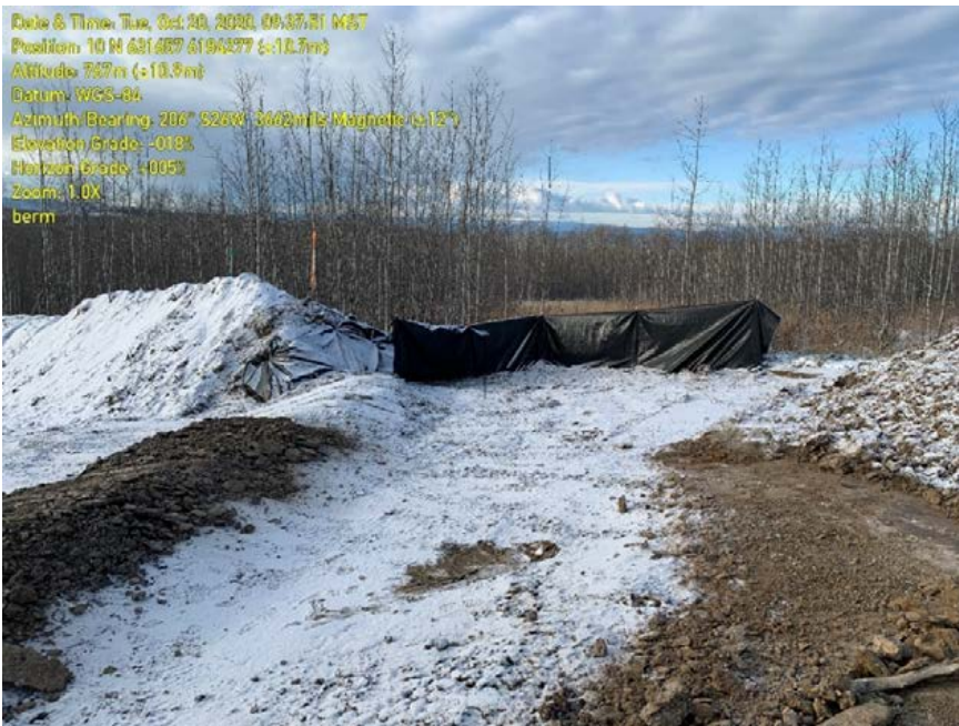
Photo 18: Sediment fence at end of berm, near KP 1+800. Potential for water to pool and escape around the edges of the sediment fence and cause erosion.
