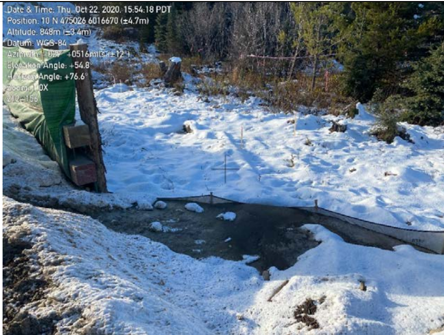
Photo 25: KP272+156. Sediment fence beside S3 watercourse overwhelmed, at risk of failing and with water passing over top of the fence.
