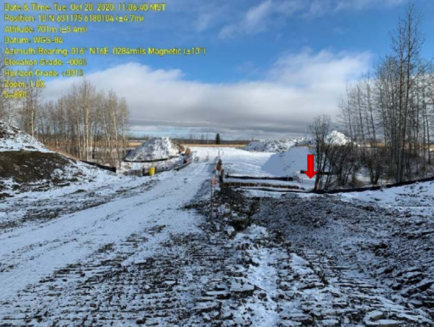
Photo 10: KP 5+890. ESC not installed to site-specific plan. Risk of sediment mobilizing to watercourse.
