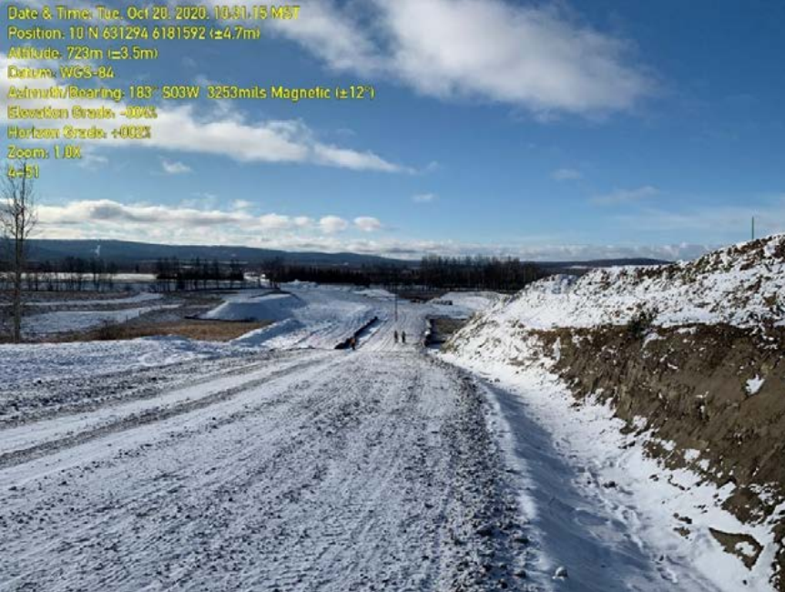
Photo 4: Ditch leading to wetland ID 0065, no ESC controls.
