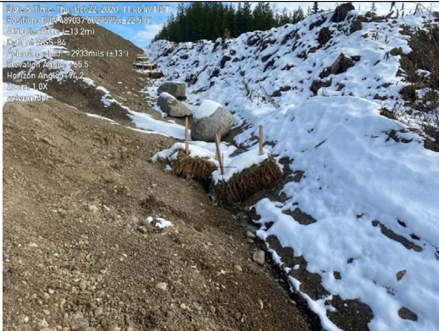
Photo 51: Incorrectly installed straw bails at the Salmon River DPI site. Bails not keyed in place and erosion has taken place beneath. Note the rocks installed upslope which are not acting as an effective ESC measure.
