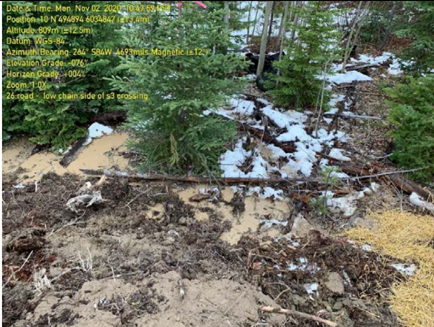
Photo 77: Opposite side of sediment fence. Sediment laden water now flowing down slope on opposite side of topsoil windrow.
