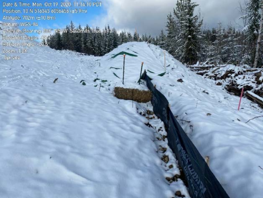
Photo 49: Ineffective straw bail not installed as required at Crooked River DPI site. Bail was not keyed into place. Water has eroded beneath the bail.
