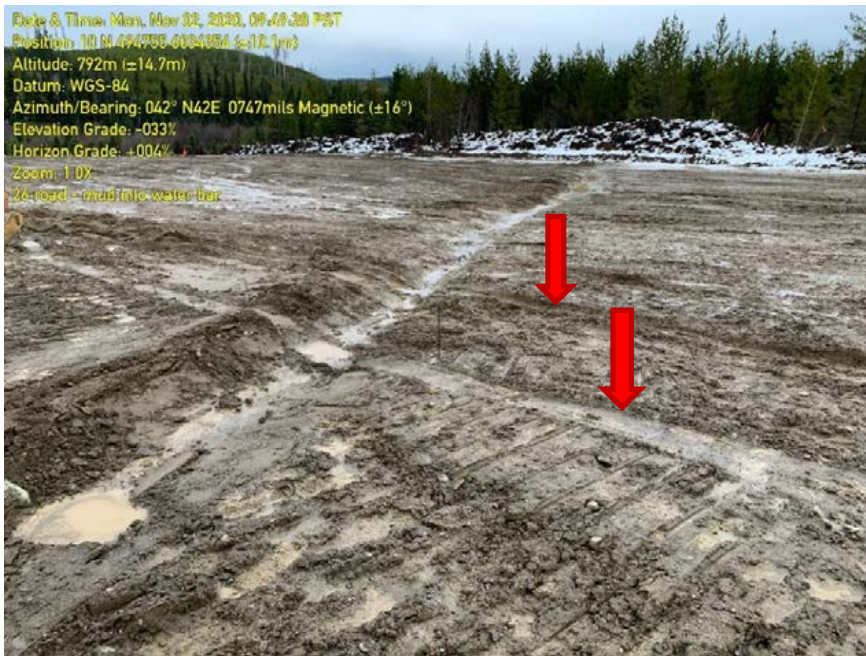
Photo 81: Upper water bar looking north, red arrow indicates tracks through water bar.
