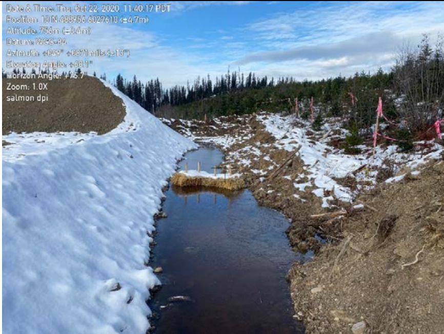
Photo 53: Non-functioning straw bails at Salmon River DPI site. Large volume of water around the straw bails.
