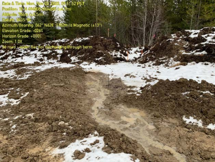
Photo 82: Exit point of upper water bar not functioning. Water continues to travel down ROW causing erosion.
