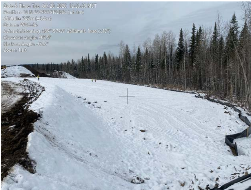
Photo 38: Work package 1, Timber Deck Area 1. Exposed material sloping towards single row of sediment fence.
