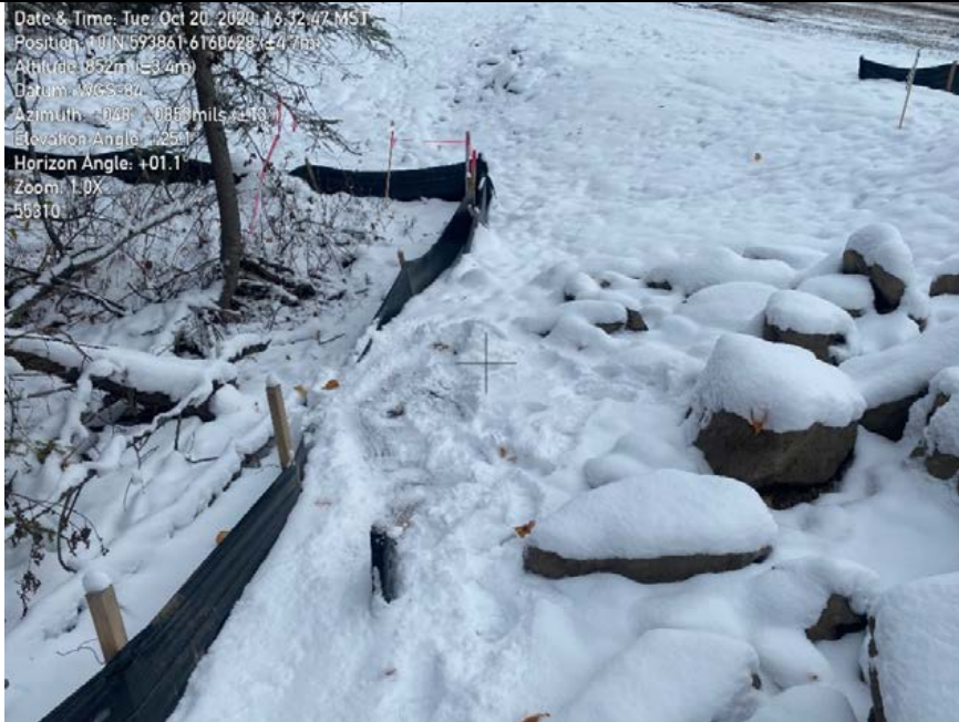
Photo 37: Same location as photo above. Sediment fence overwhelmed with material from the ROW. Material discharging off site.
