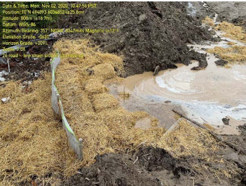
Photo 76: Gap in topsoil windrow. Sediment laden water passing through sediment fence and straw.
