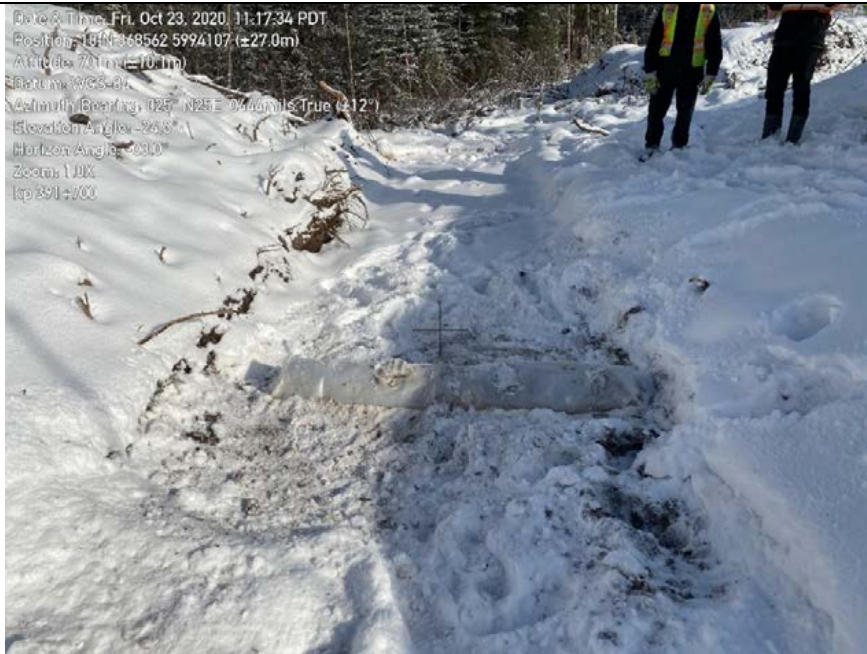
Photo 57: Work package 3. Check dam of sandbags covered with poly installed in ditch. Measure does not extend across ditch; flow can escape around the structure. Not effective. Exposed area seen in Photo 47 above is designed to drain to this ditch and then into the vegetated area beyond the right of way.
