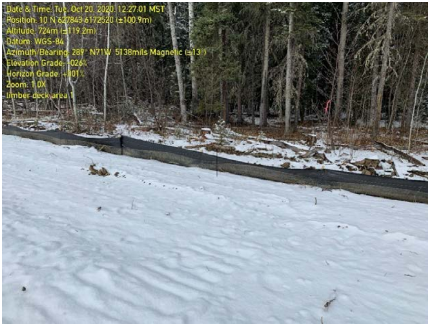
Photo 39: Work package 1. Low point along sediment fence in Timber Deck Area 1. Staining on sediment fence showing how high sediment build up in this area has been previously.
