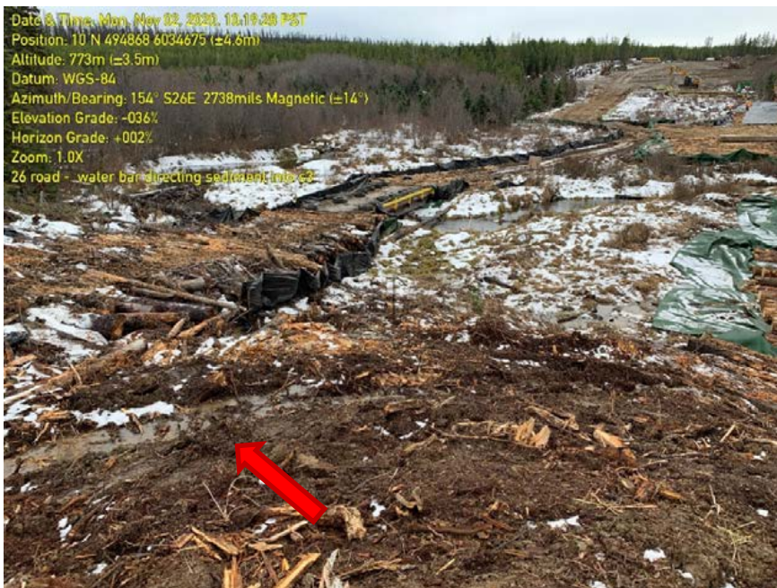
Photo 67: WC272, Low chain looking towards high chain. ESC measures along banks of stream are limited to incorrectly installed and unmaintained sediment fence, increasing risk of sediment transport to fish-bearing watercourse. Red arrow showing erosion and sediment transport towards and into fish-bearing stream.
