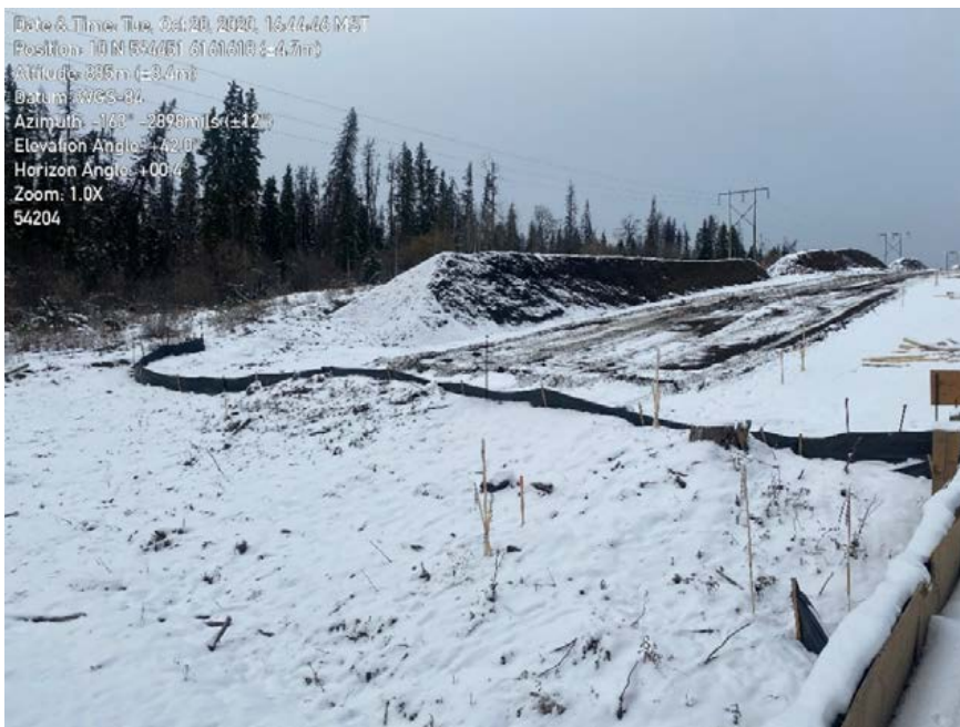
Photo 34: Work package 1, KP54+204. Right bank approach to S3 stream is roughly 170 m long of exposed material. Single row of sediment fence at the base of the slope as ESC measure.
