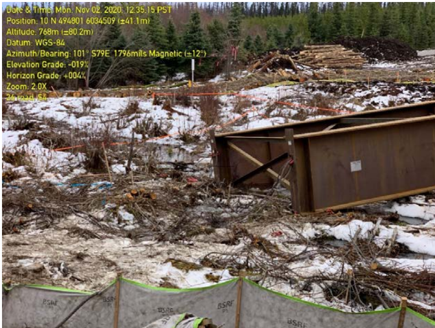
Photo 87: Steel girder dropped into S4 channel. Upstream looking downstream.
