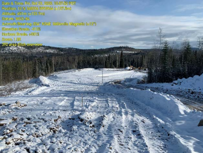
Photo 47. Work package 3, exposed soils on right of way draining towards single confined area. See Photo 57 below for image of where this material is designed to drain to.
