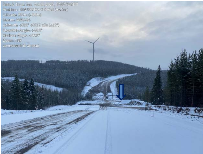
Photo 40: Work pack 1, exposed soils from right of way draining down slope towards S6 stream feature. Blue arrow roughly indicating location of stream.
