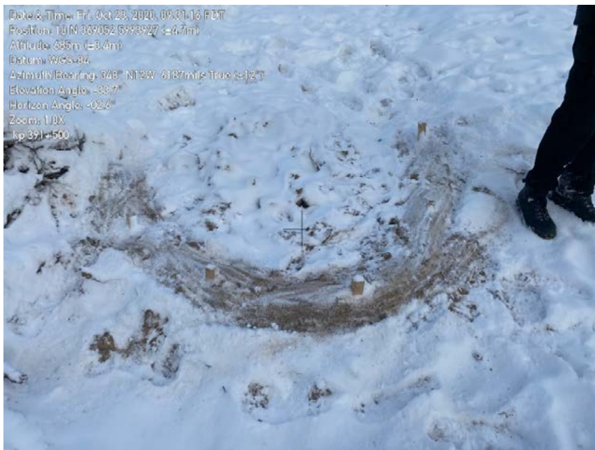
Photo 56: Work package 3. Straw roll keyed in too deep, limited catchment area as a result.
