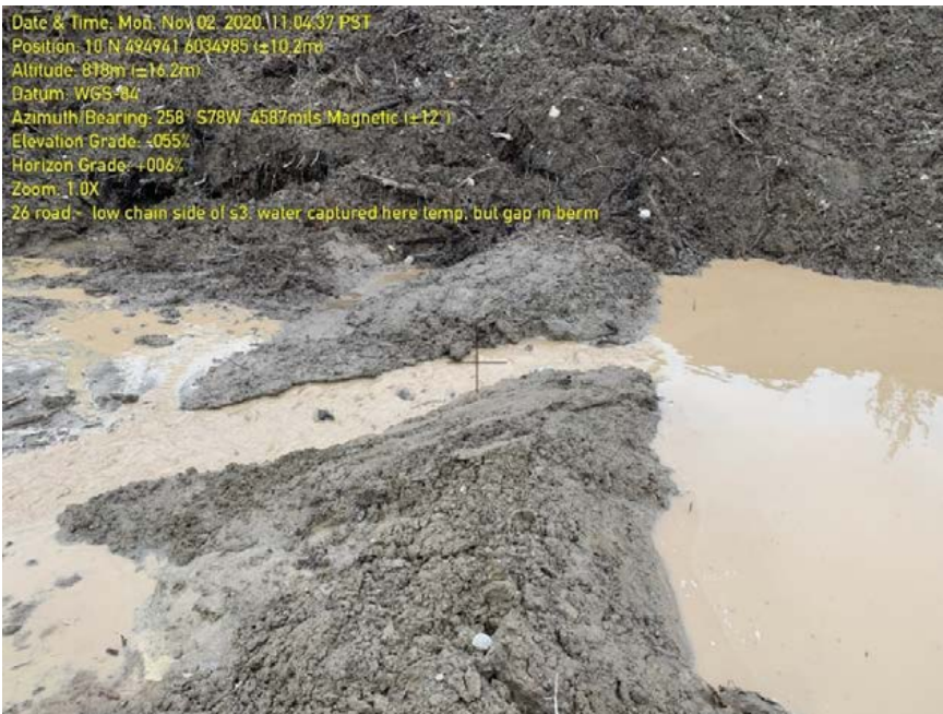
Photo 73: Notch in berm causing water to continue to travel down slope towards fish-bearing stream.
