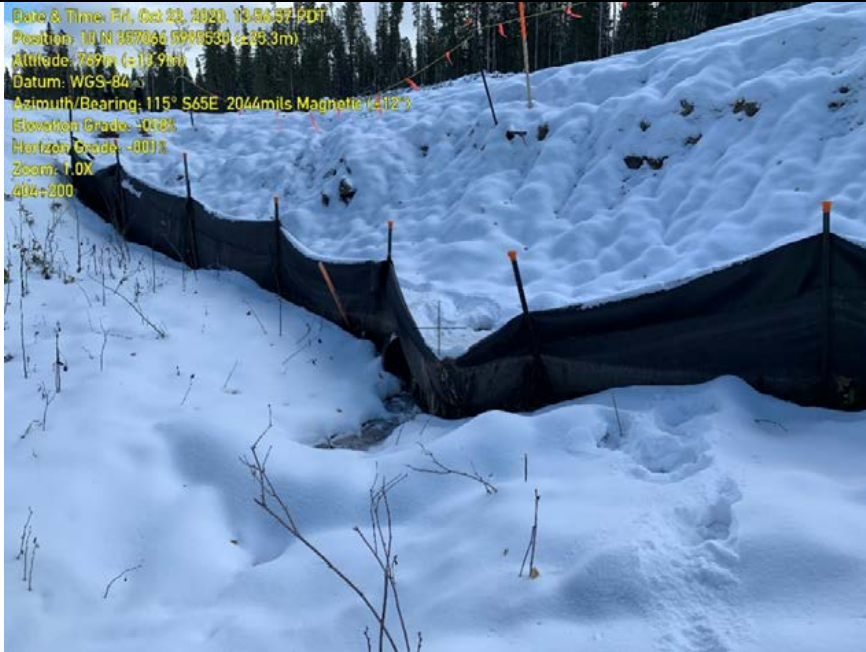
Photo 29: Material from bridge approach overwhelming sediment fence. Fence at risk of failing. Wetland (W2) at this location.
