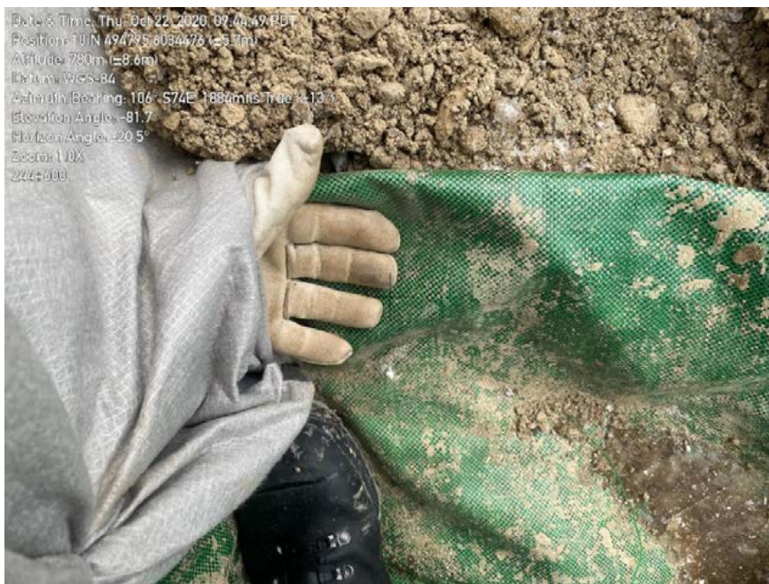
Photo 26: Sediment fence adjacent to watercourse not fastened correctly to another length of sediment fence. Large gap allows water to flow beneath.
