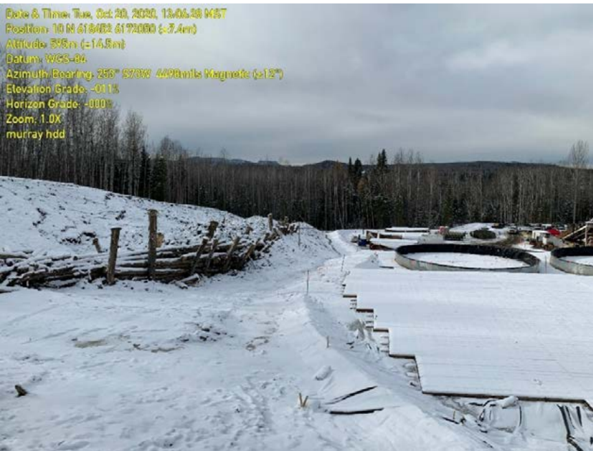
Photo 11: KP 24+550, Murray HDD site. Drainage channel on left side of pad. Continuous ditch line leading down slope with no ESC measures within ditch.
