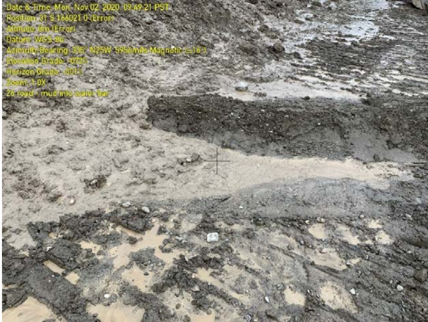
Photo 80: Soil stockpile material sloughing into water bar.
