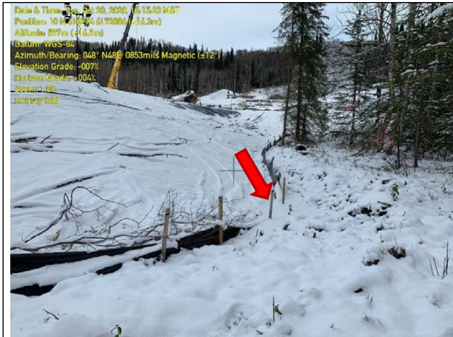
Photo 12: Red arrow indicating failed sediment fence at base of drainage ditch on left side of Murray HDD pad.
