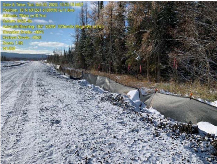
Photo 16: Wetland ID 040, failing sediment fence.
