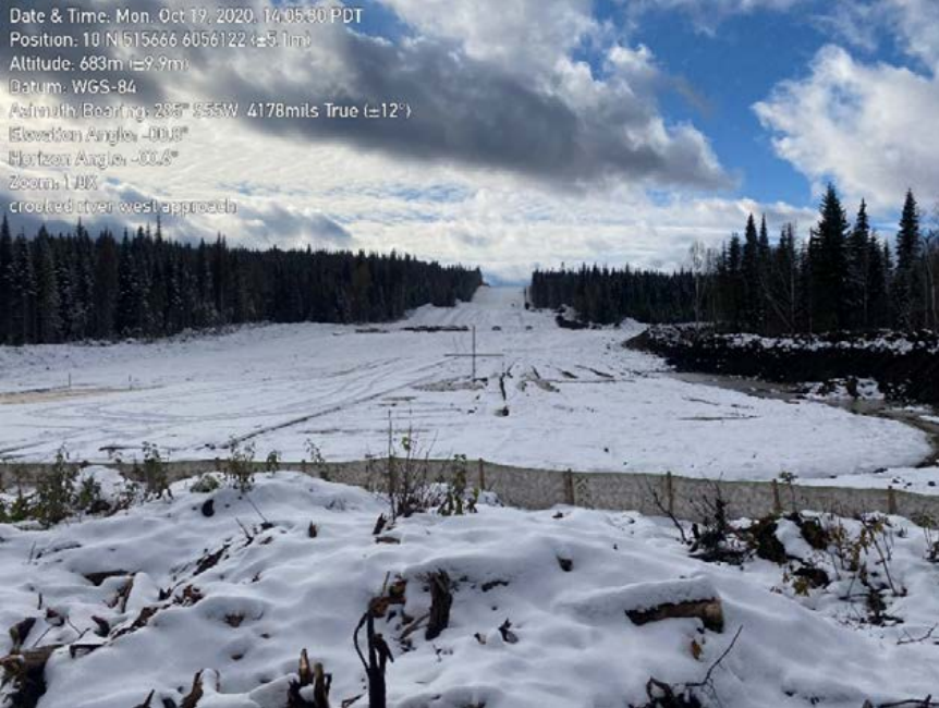
Photo 45: Work package 2. Right bank side of Crooked River. Exposed right of way with limited erosion and sediment controls in place. Approach is roughly 600 m long x 80 m wide with the cleared laydown measuring approximately 130 m long x 125 m wide. Both upslope areas report to the base of the slope adjacent to the Crooked River. See photo below for different perspective of where this location drains to.
