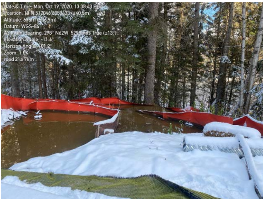
Photo 22: Sediment fence installed across a channel downstream of culvert outlet at 7 km on 21a road. Crooked River in background downslope of this location.
