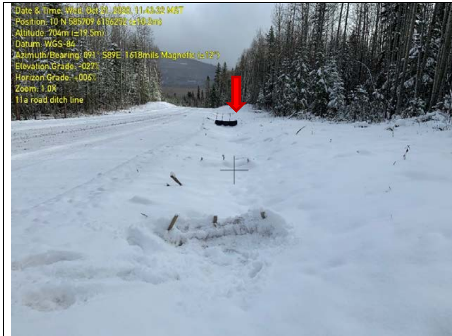
Photo 19: 11a road ditch line, example of sediment fencing installed in ditch line. Not a recommended use for sediment fencing; will increase erosion in ditch.
