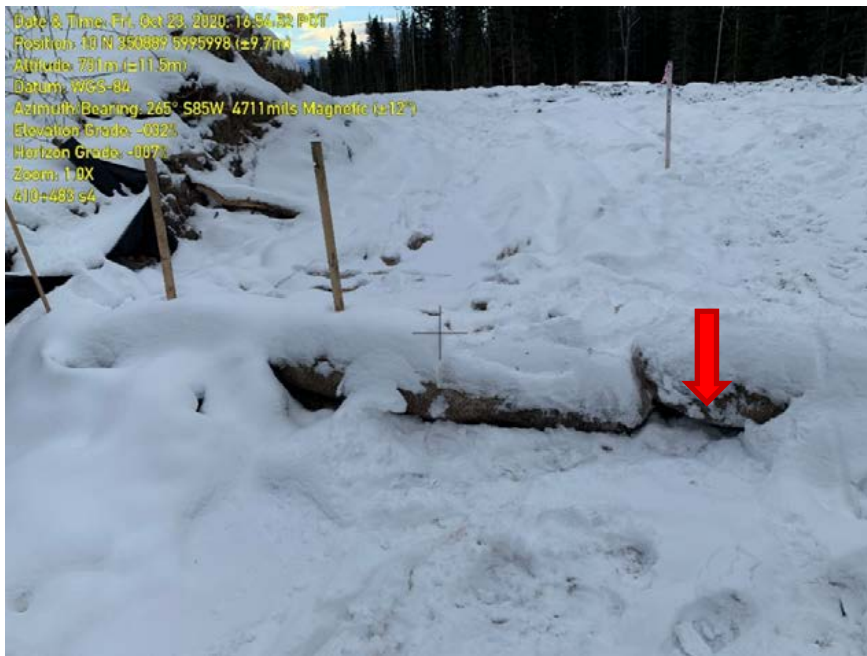
Photo 58: Work package 3. Straw rolls not keyed into place; arrow indicating gap beneath the straw roll.
