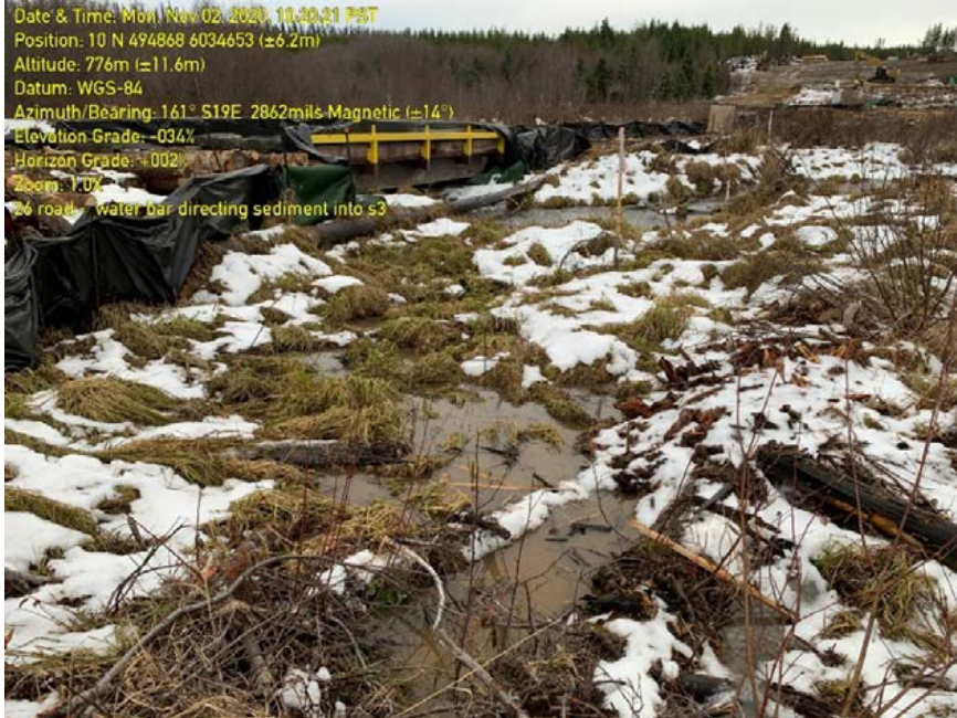
Photo 68: WC272, no ESC measures where turbid flow from erosion on right-of-way entering fish bearing watercourse.
