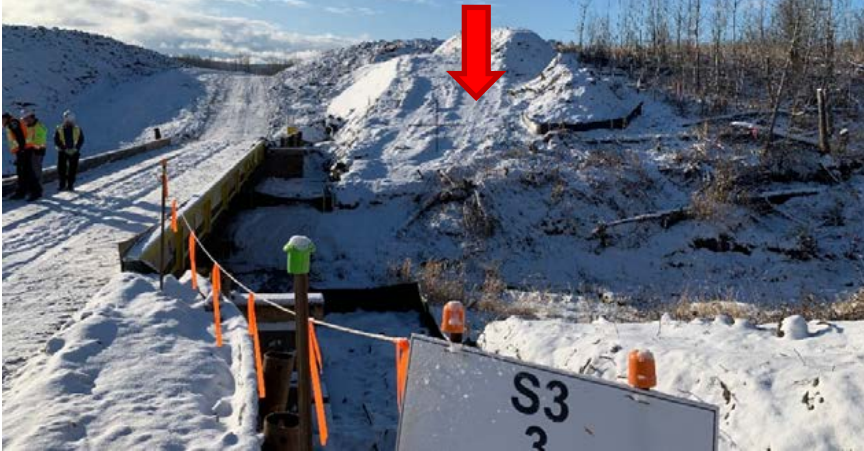
Photo 8: KP 5+607 with disturbed and exposed slopes leading to fish-bearing stream (S3).
