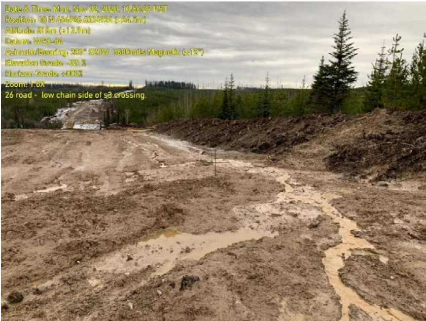
Photo 2: Exposed right of way near KP244. Lack of winterization following stripping has caused erosion on the right of way leading to impacts to a fish-bearing stream.
