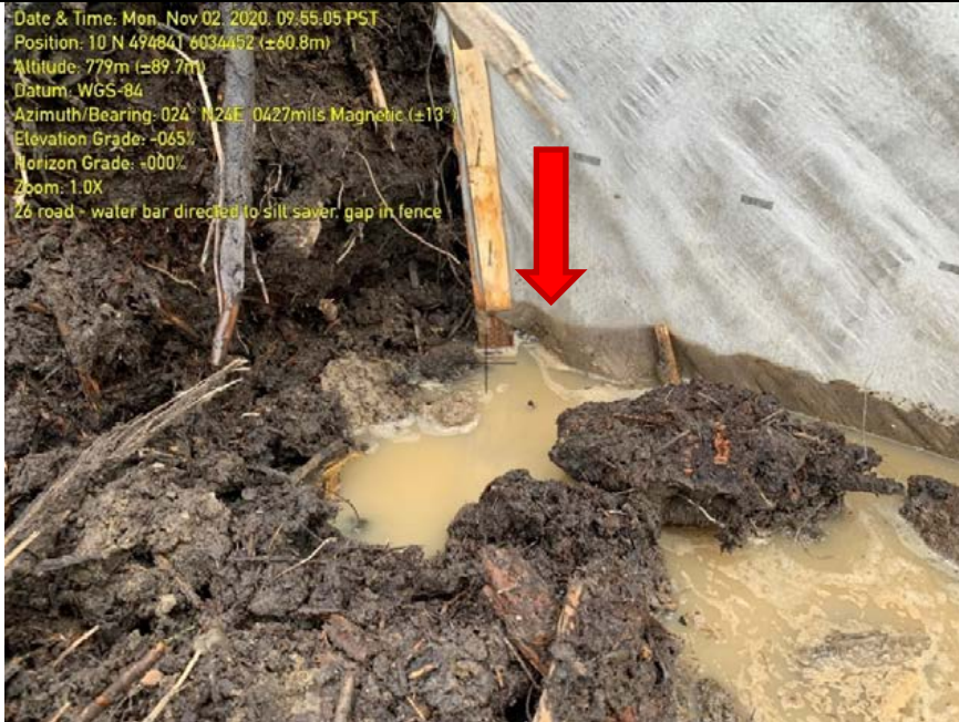
Photo 84: Gap in sediment fence at end of water bar.
