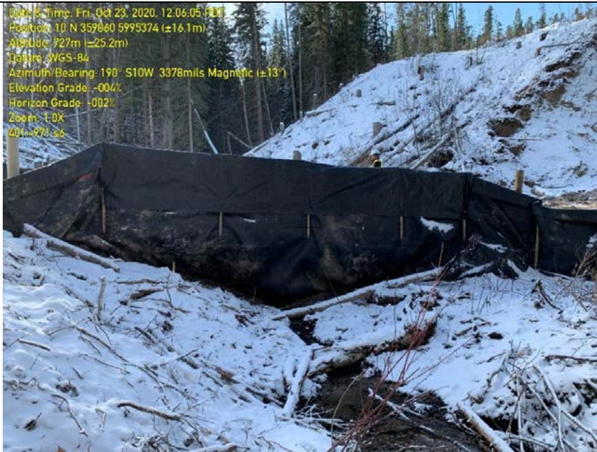
Photo 61: Work package 3. Geotextile fabric from bridge crossing sagging into watercourse.
