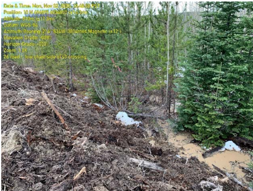
Photo 78: Opposite side of sediment fence. Sediment laden water now flowing down slope on opposite side of topsoil windrow.
