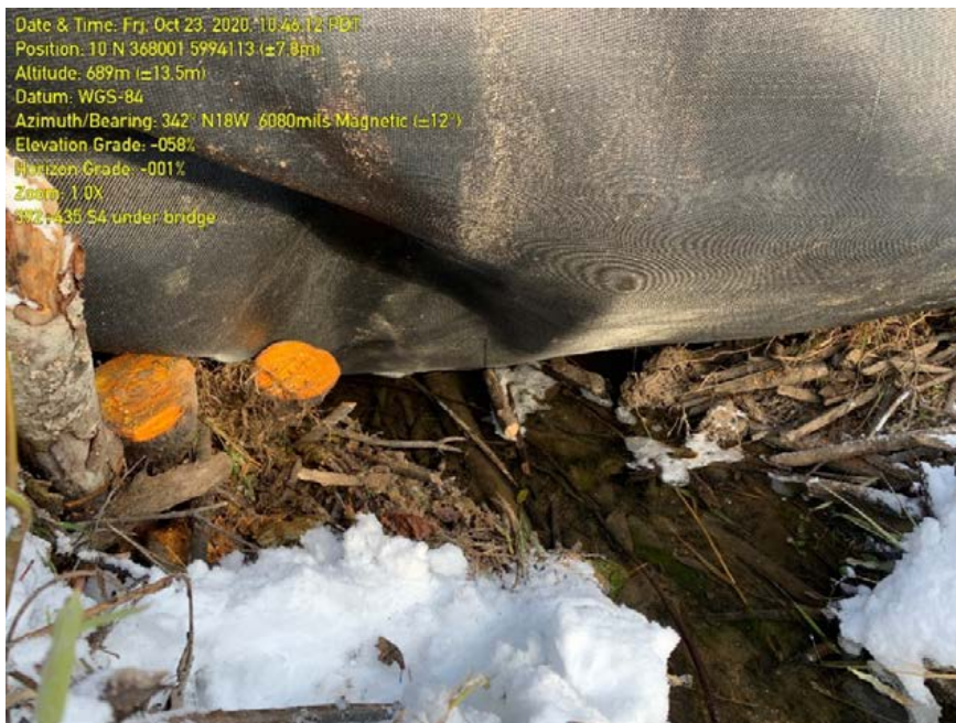
Photo 60: Close up of geotextile from bridge over S4 stream at KP392+435 sagging into channel.
