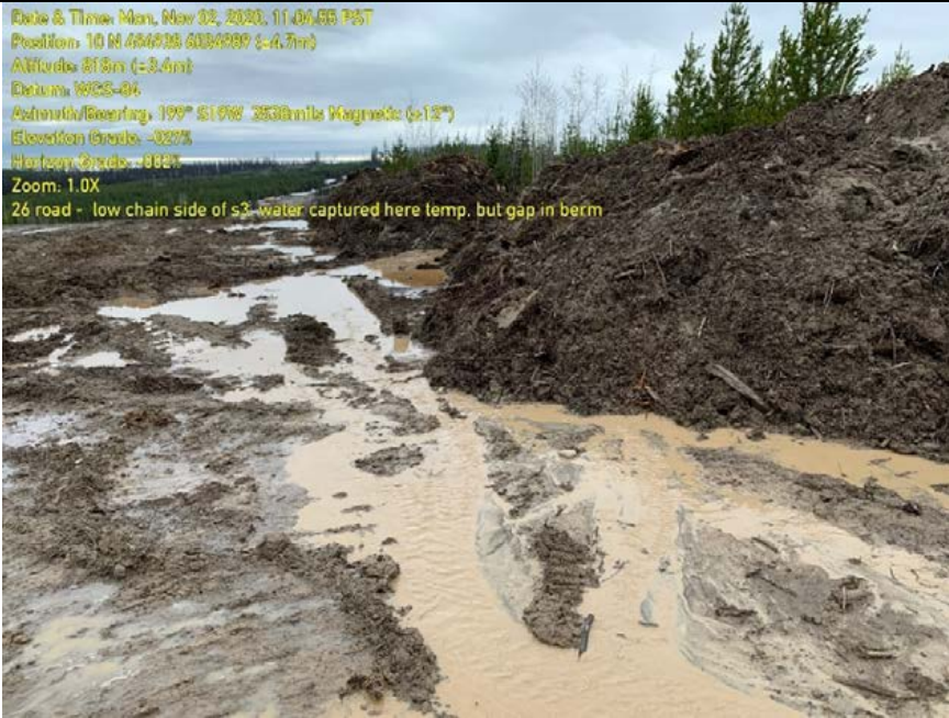
Photo 74: Flow down slope after the berm.
