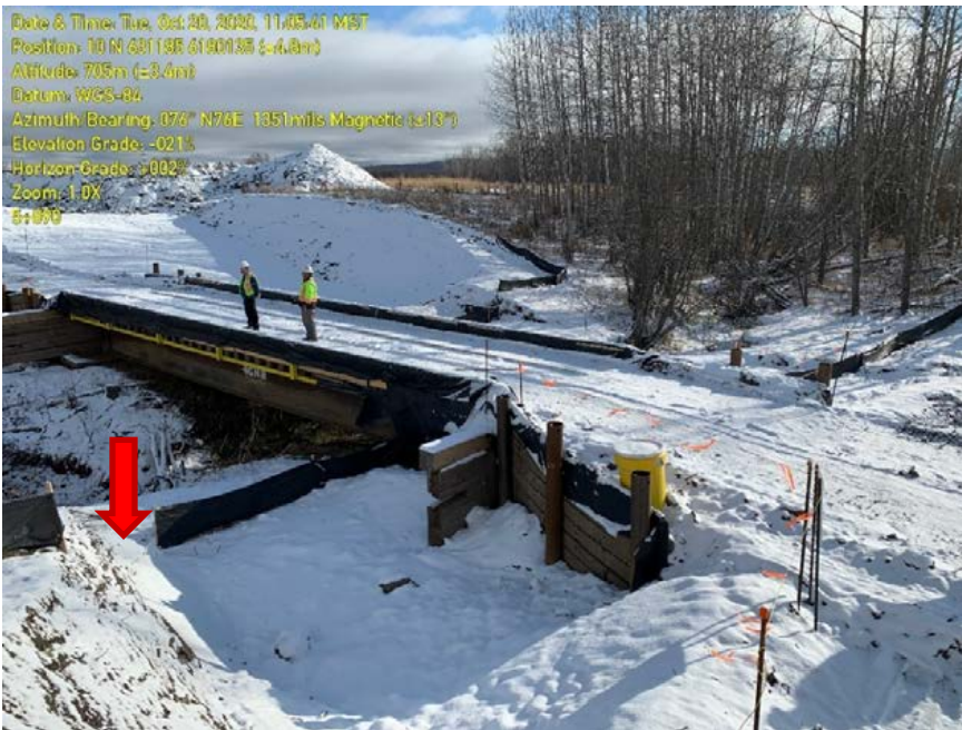
Photo 9: KP 5+890. ESC not installed to site-specific plan. Risk of sediment mobilizing to watercourse.
