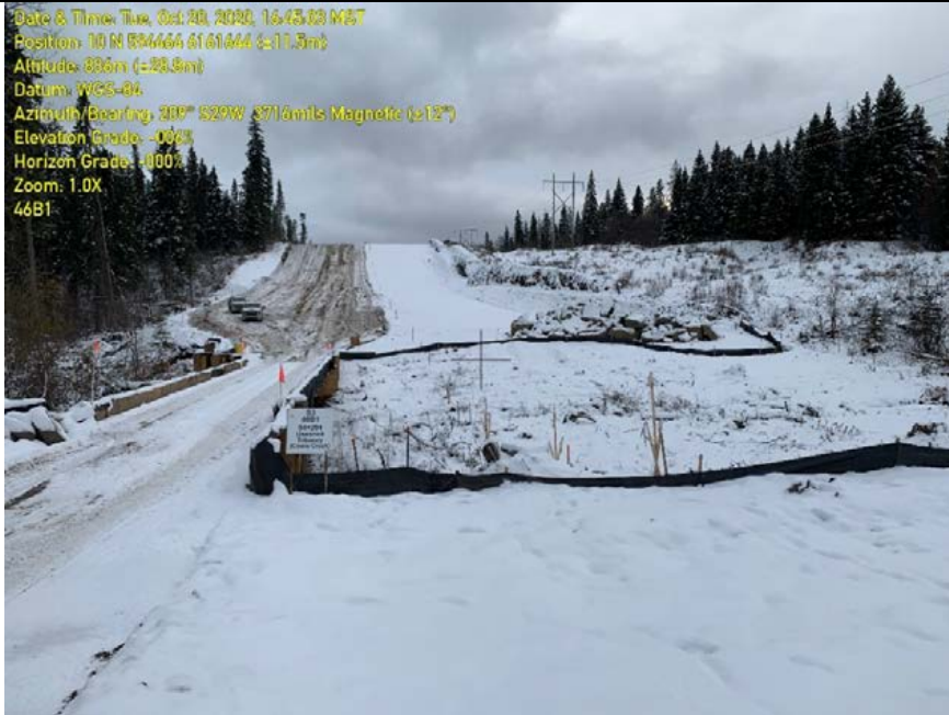
Photo 33: Work package 1, KP54+204. Exposed right of way drains to single row of sediment fence adjacent to S3 stream.
