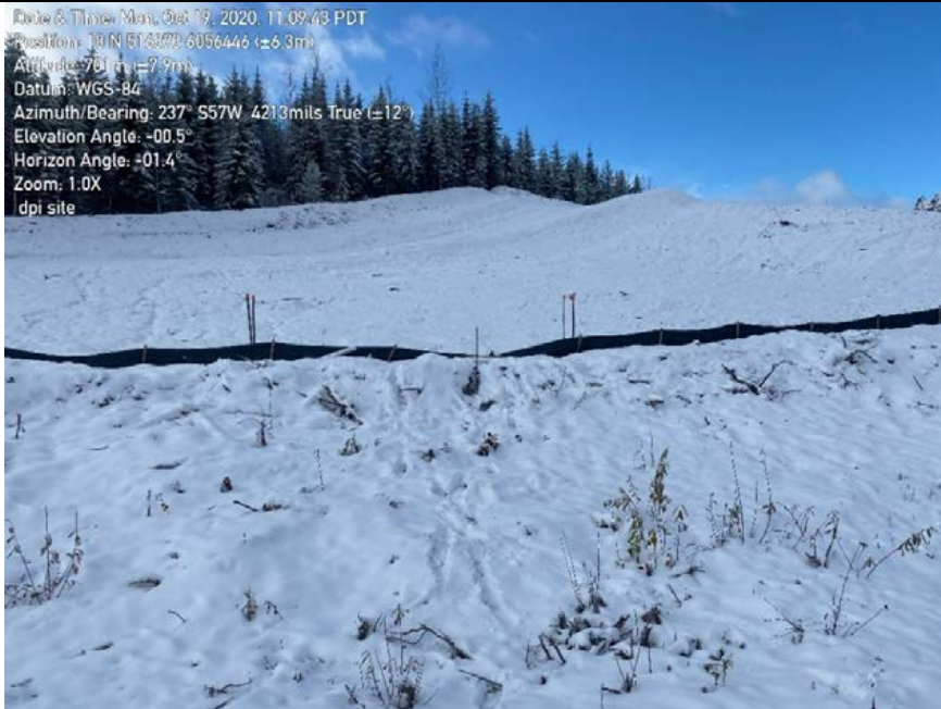
Photo 41: Work package 2. At the left bank side of Crooked River DPI site, low-chain looking towards high-chain. Long exposed slope draining to single row of sediment fence.
