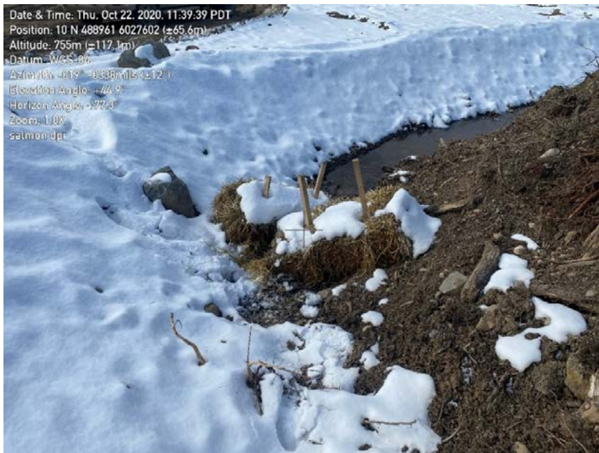
Photo 52: Incorrectly installed straw bails at the Salmon River DPI site. Water has eroded beneath the structures.
