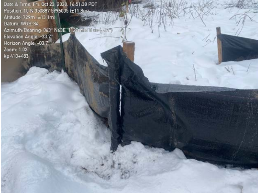
Photo 31: Gap left between sections of sediment fence. Water can pass through this gap. This incorrect installation practice was commonly seen including at KP402+803, 404+200 and 408+592.
