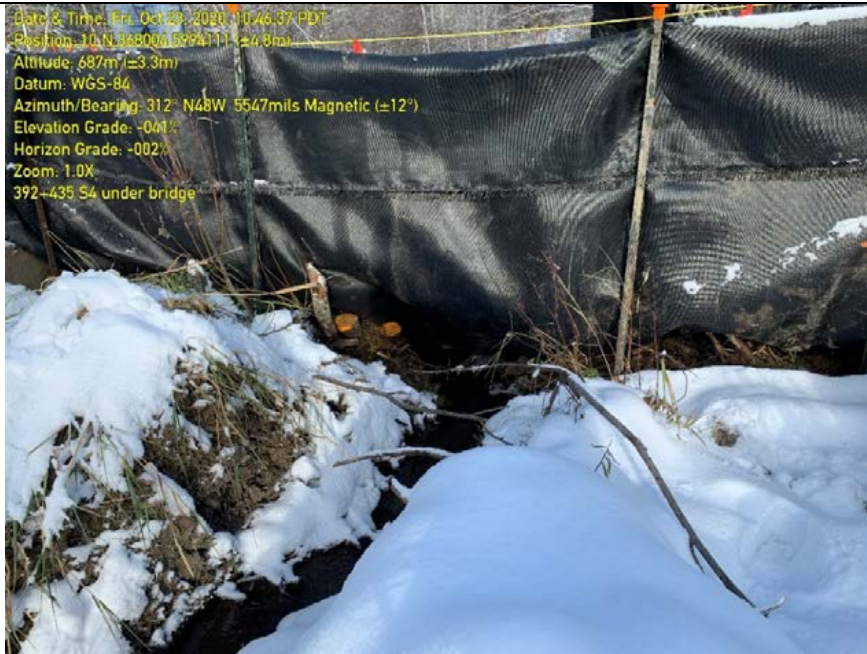
Photo 59: Geotextile from bridge over S4 stream at KP392+435 sagging into channel.
