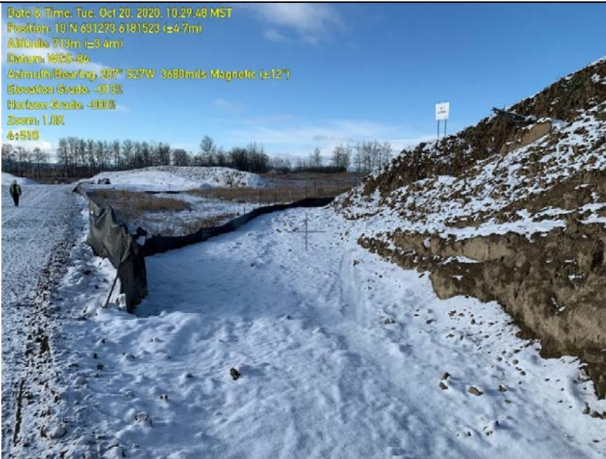
Photo 6: KP 4+518, bottom of ditch, sediment deposition adjacent to wetland ID 0065.
