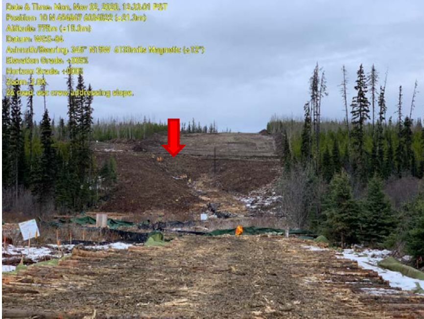
Photo 86: Arrow indicating crew members installing ESC measures on slope to S3 stream.
