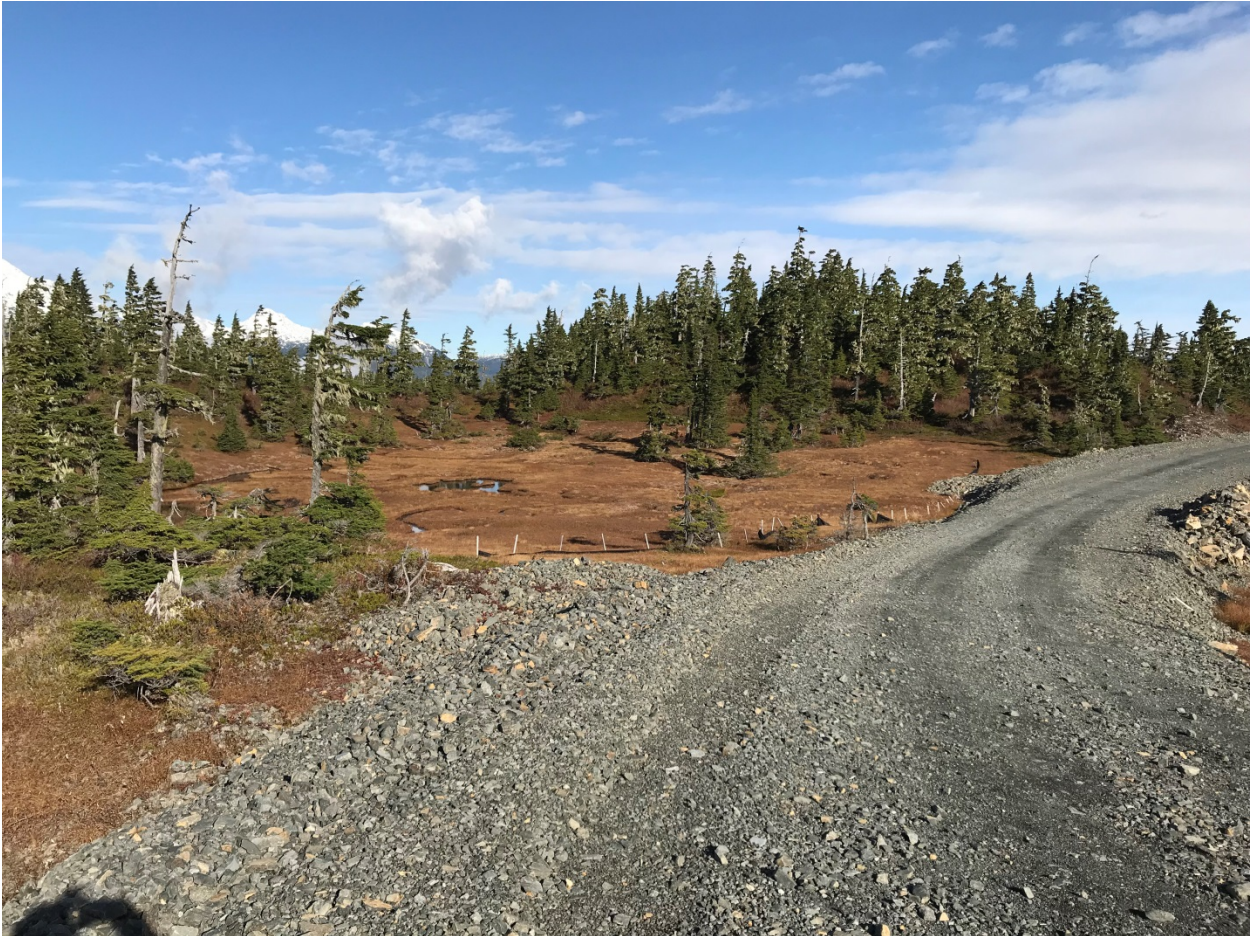
Figure 4: On site Mine access road to the Plant Site Area. Constructed to accommodate two way light vehicle traffic and concentrate haulage to and from main Mine site area.
