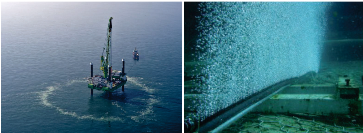
Figure 2. Example of air bubble curtain. (Left): Active air bubble curtain around pile driving activities. (Right): Tubing for an active air bubble curtain.
